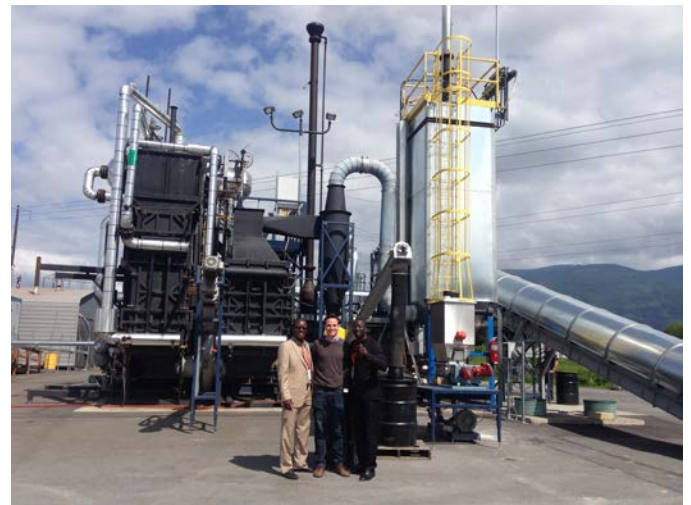
DELVIC Representatives with a JB Engineer, Standing in front of the S200 Unit at Janicki Bioenergy Headquarters
