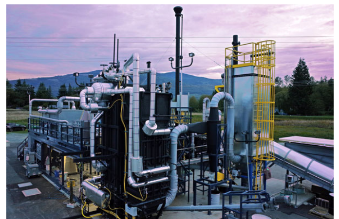
Boiler and baghouse side of the S200
