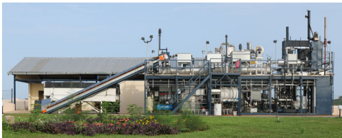
Dakar JOP pilot plant
